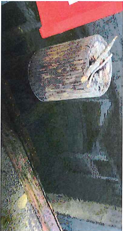
TIMBER PILE CONDITION
