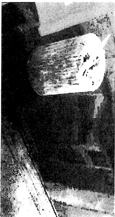
TIMBER PILE CONDITION
